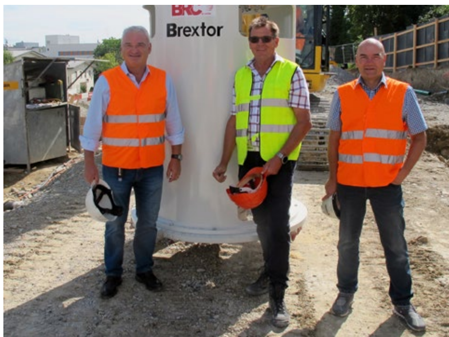
The Aregger company is using the Brextor for the first time in Opfikon. Photo: Entrepreneur Hans Aregger, Brextor inventor Alois Portmann and Urs Odermatt, Head of Civil Engineering Aregger (from left).
