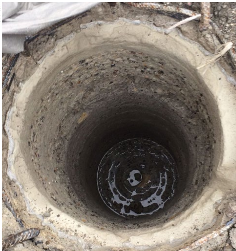
Foreign material and dirt in the concrete impair the static function of piles. With the inner milling cutter, piles can be bored out to a depth of six metres for renovation work, so that a second pile cage can be concreted in.
