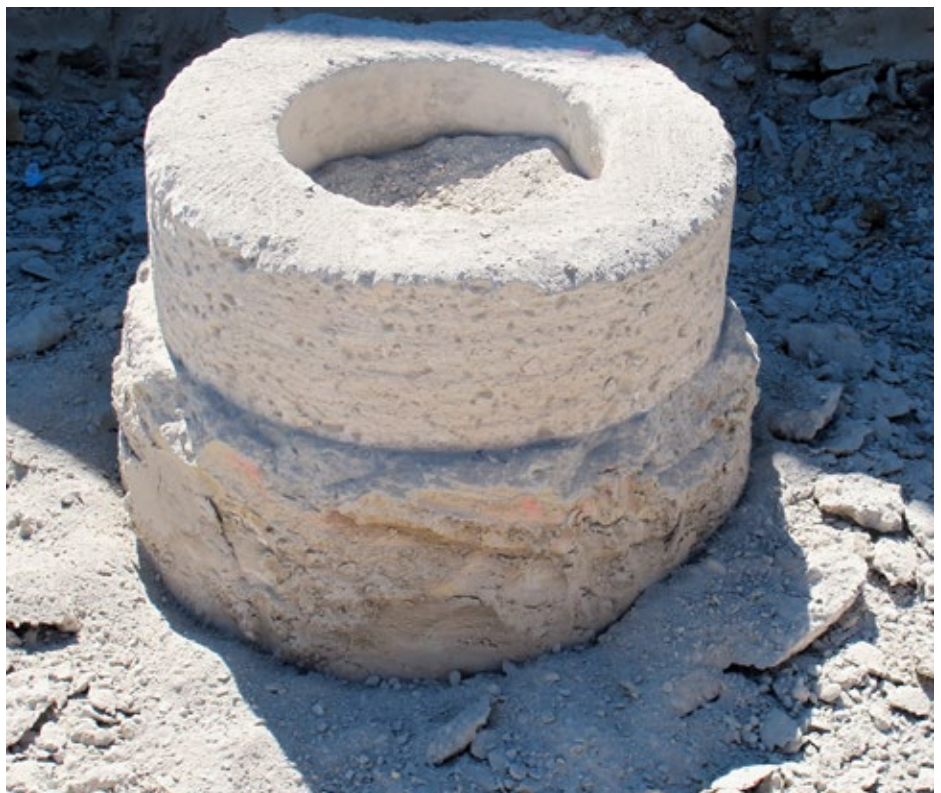
The result after the second phase of pile head processing is a hollow cylinder, which still contains the reinforcing bars. These are then exposed.
