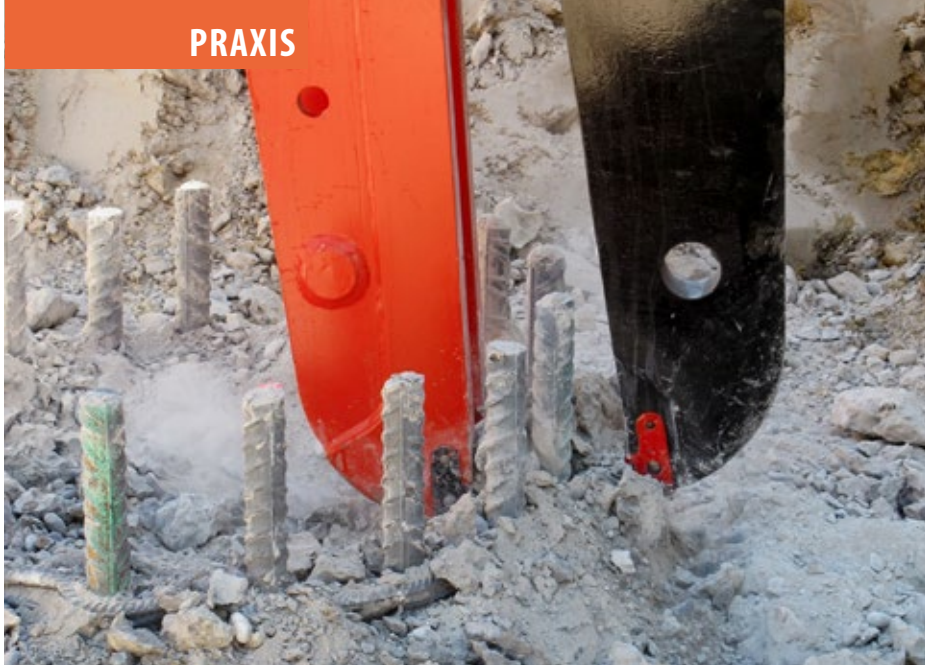
The biter exposes the reinforcing bars (phase 3). Any residue on the concrete surface and between the rebars is removed with an electric hammer.
